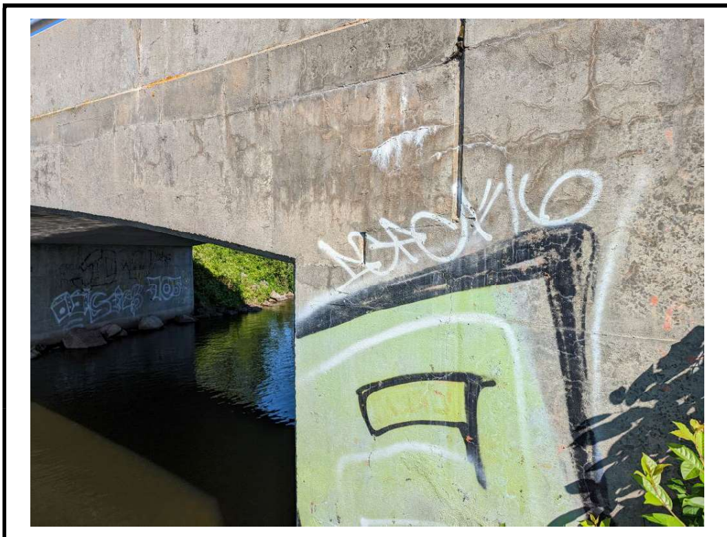
Photo 14 Narrow cracks, damp stains with efflorescence, & graffiti on southeast wingwall.
