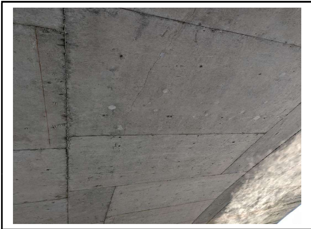
Photo 16 Narrow longitudinal cracks noted with origins at abutment wall
