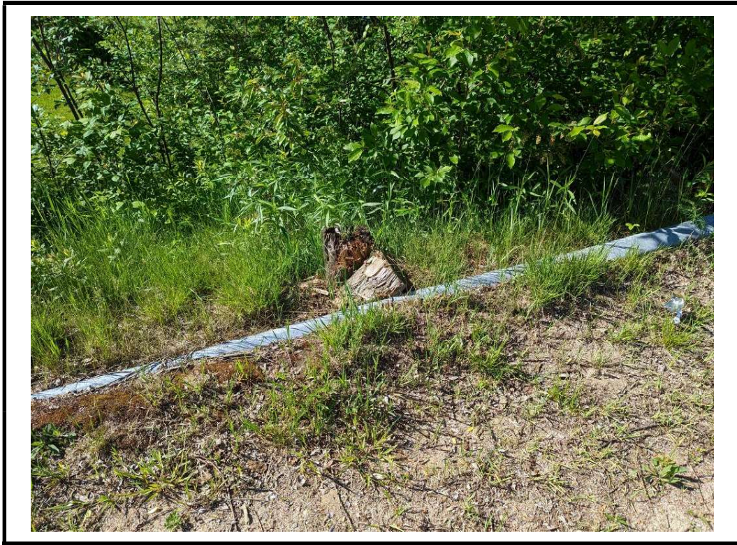
Photo 7 Typical buried end treatment and rotted post at southeast corner
