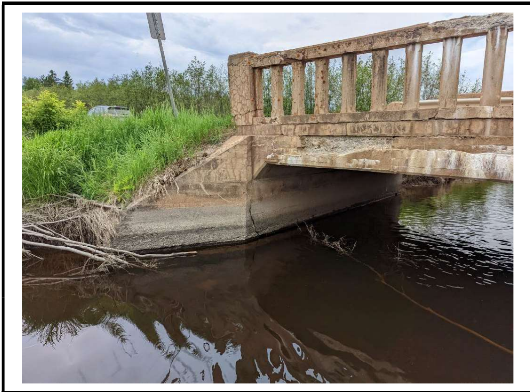
Photo 9 Severe spall and cracks with efflorescence noted on south fascia
