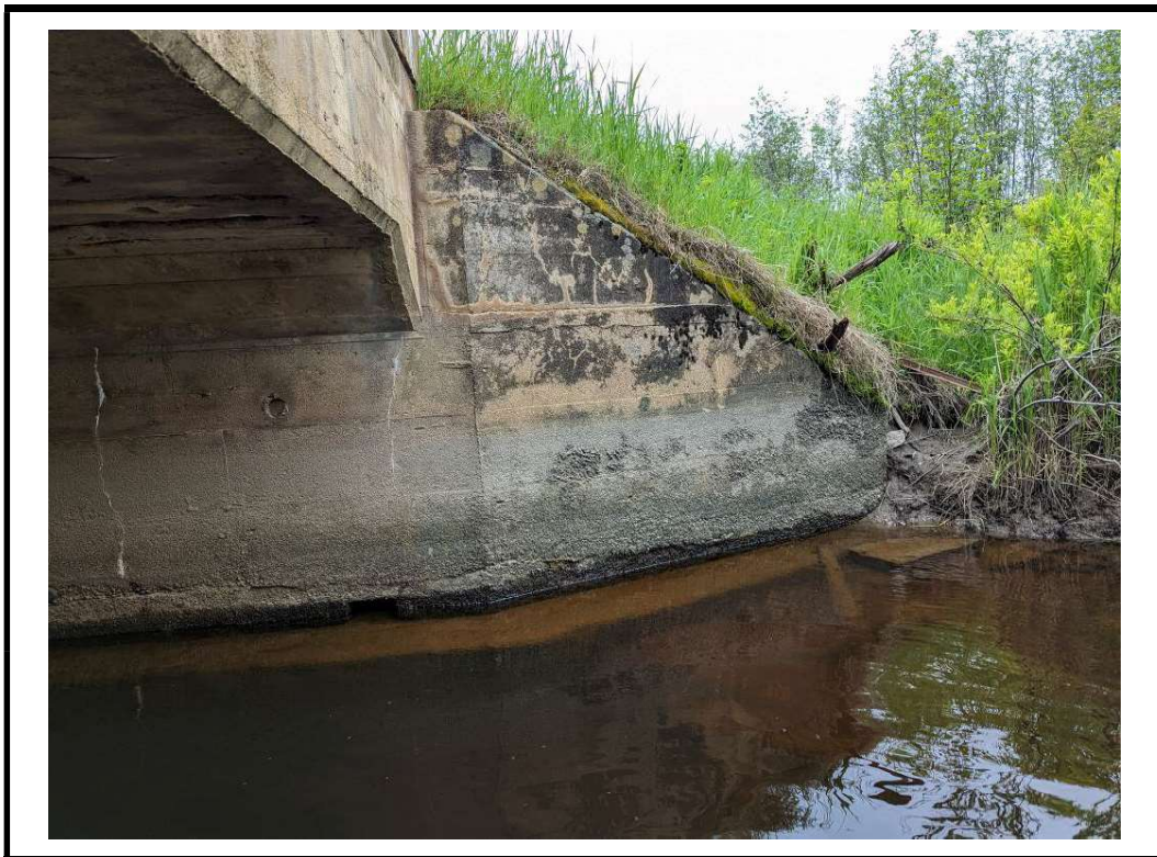
Photo 12 Narrow cracks with efflorescence noted on northwest wingwall.
