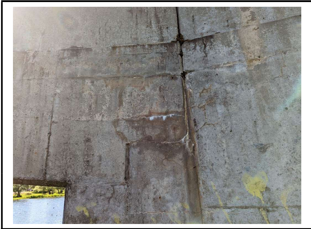
Photo 13 Narrow longitudinal and transverse cracks and damp stains on fascia.
