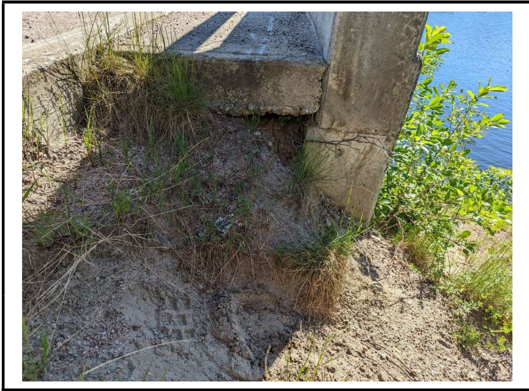
Photo 17 Minor washout noted at southwest corner near deck end
