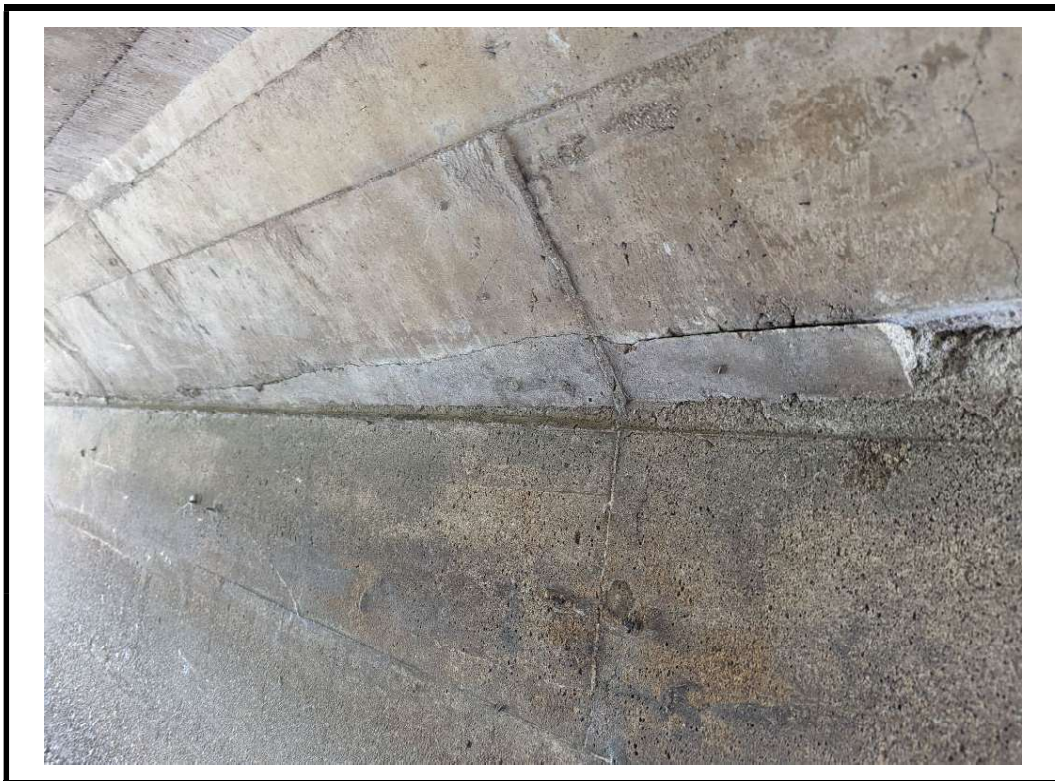
Photo 14 Small spall and longitudinal cracks noted at haunches
