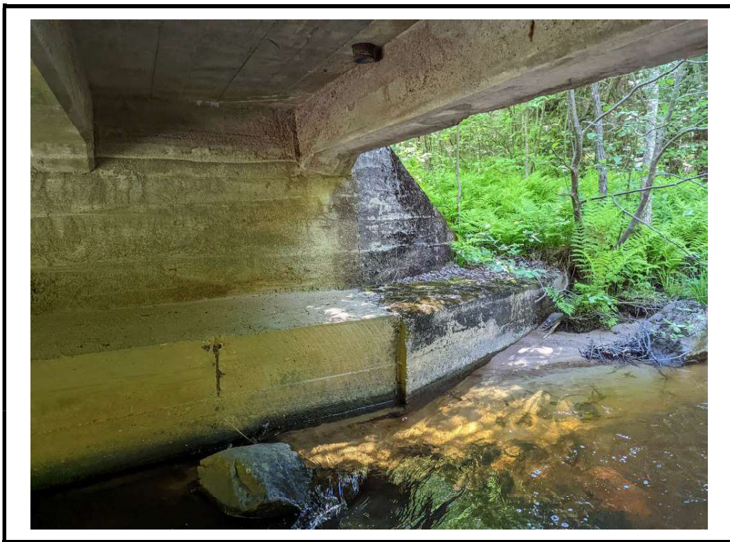
Photo 14 Spall with exposed corroded reinforcing steel on abutment wall
