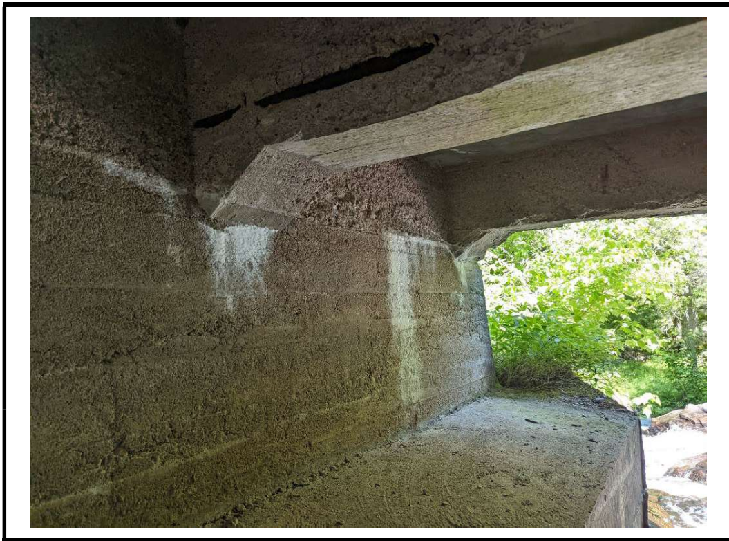
Photo 15 Moderate scaling and efflorescence stains noted on abutment wall
