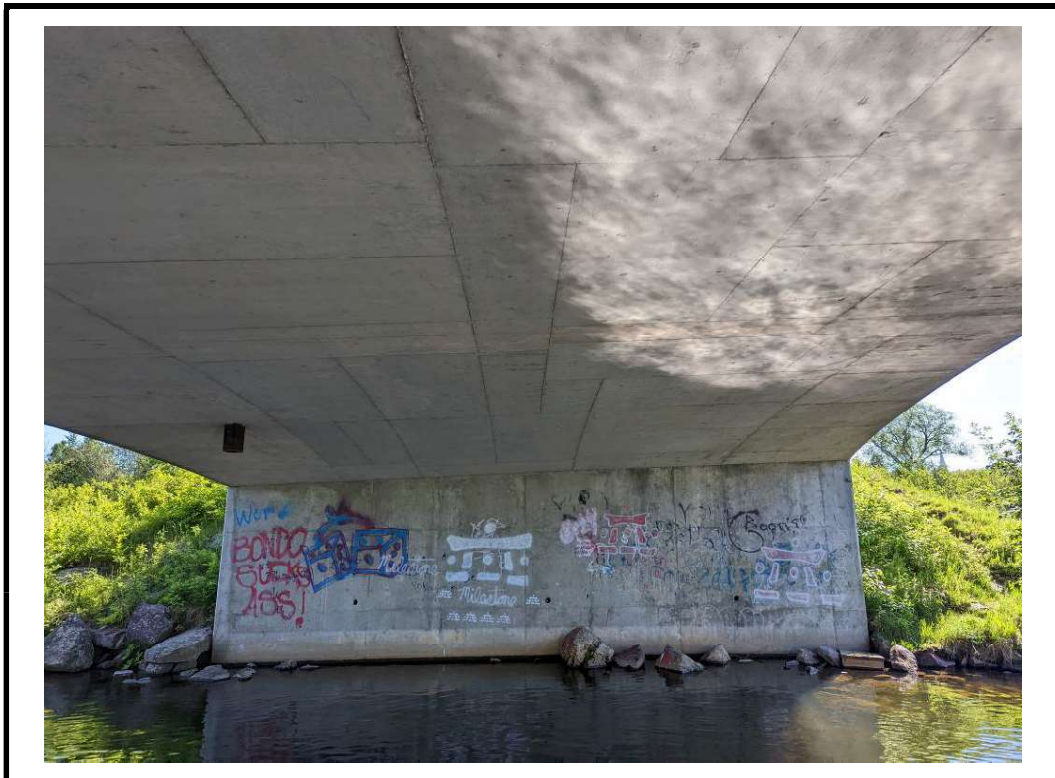
Photo 20 Narrow full length vertical cracks and graffiti noted on abutment walls (Typical)
