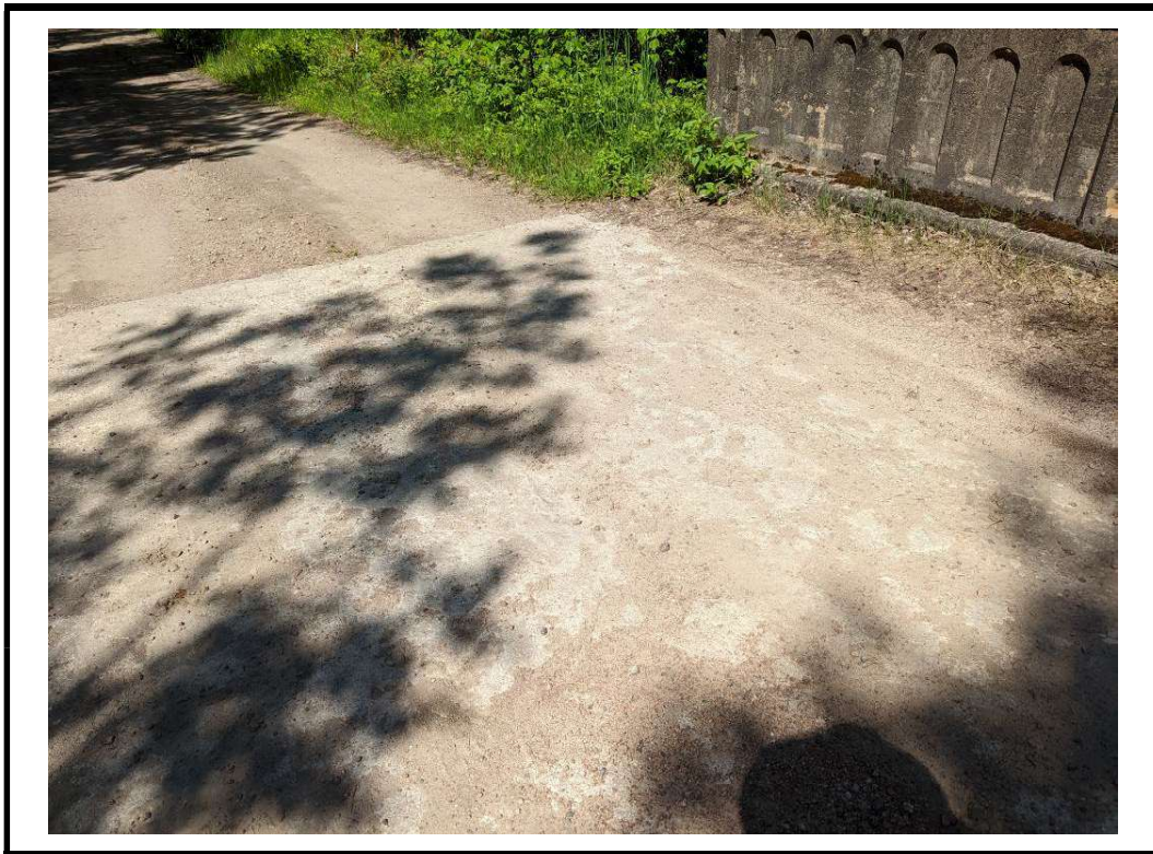
Photo 8 Moderate scaling, small spalls and dirt accumulation on exposed deck top.
