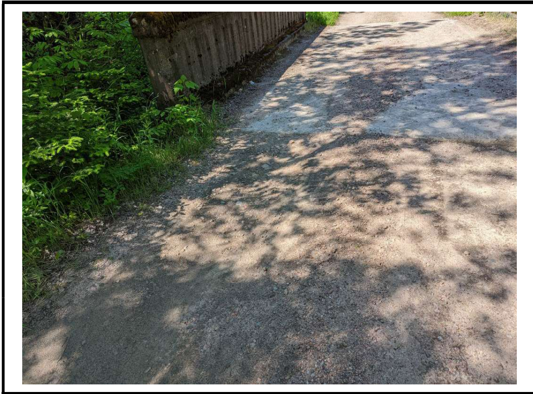
Photo 7 Large potholes on east approach.
