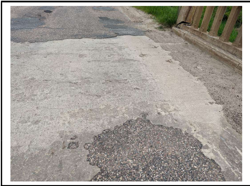
Photo 11 Minor scaling, medium spall and debris noted on deck top
