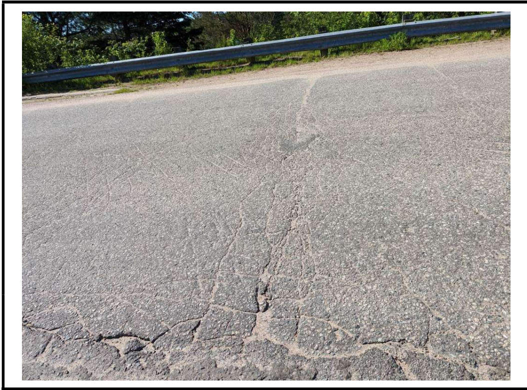
Photo 9 Medium transverse cracks with potholes in west approach
