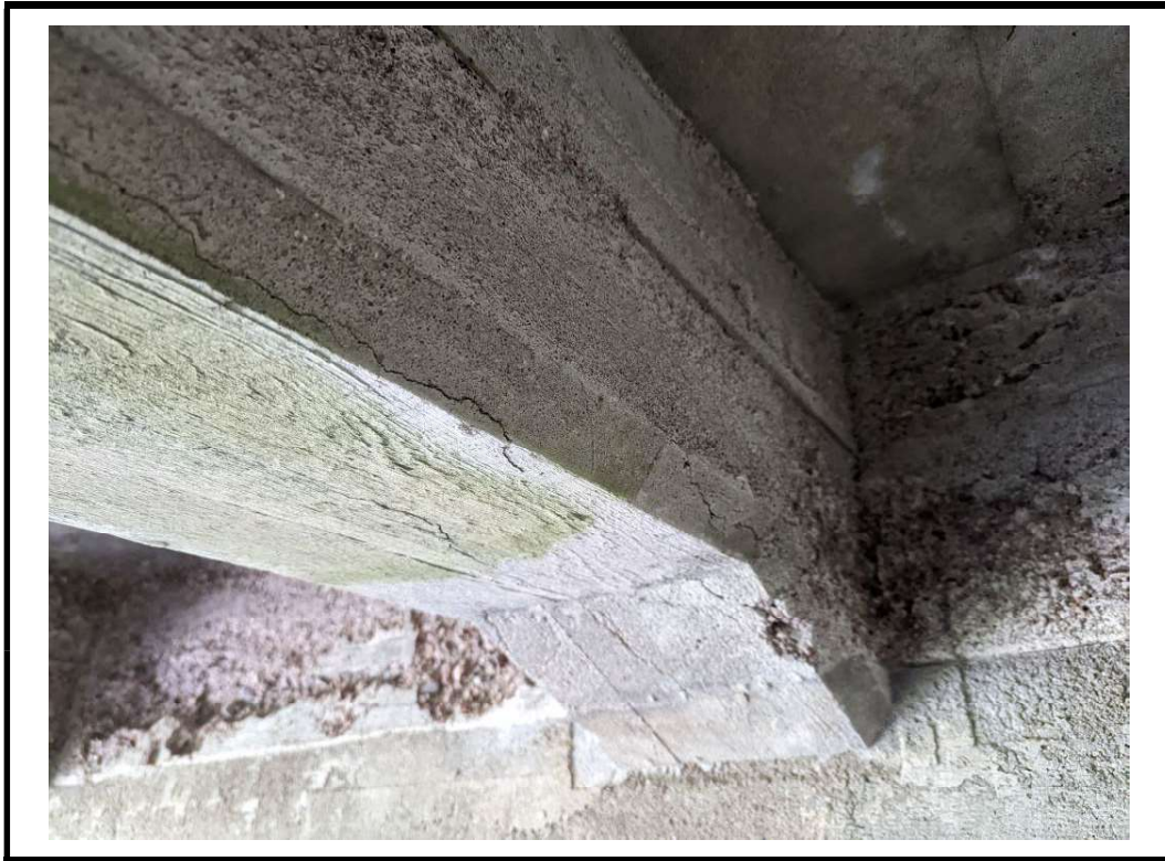
Photo 17 Spall and longitudinal cracks noted on girders
