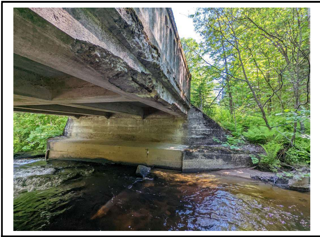
Photo 11 Spalls with exposed corroded reinforcement on face of exterior girder
