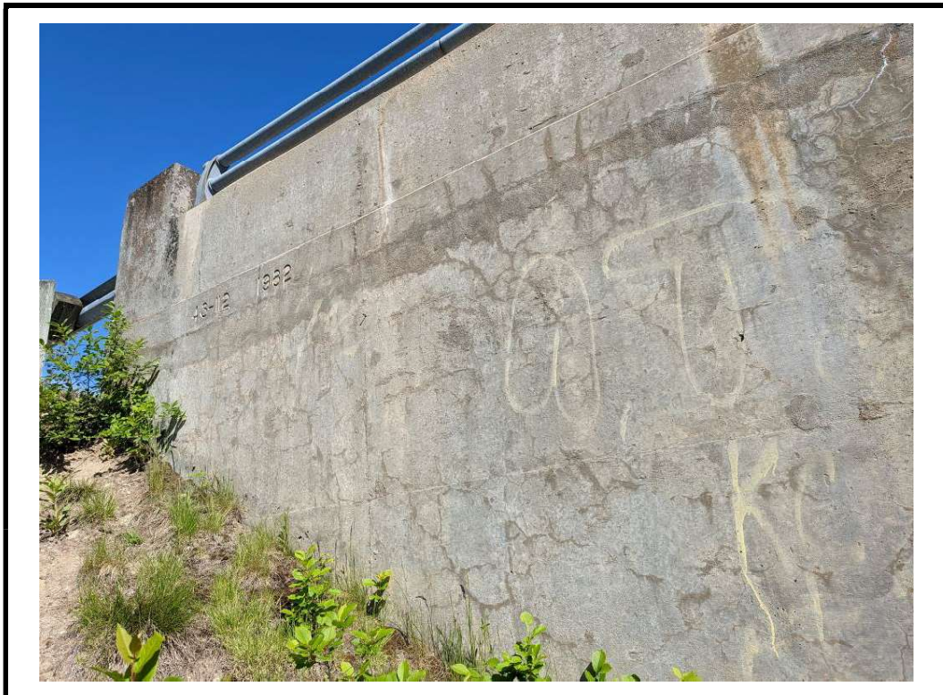
Photo 18 Typical southwest wingwall with graffiti and damp map cracks throughout
