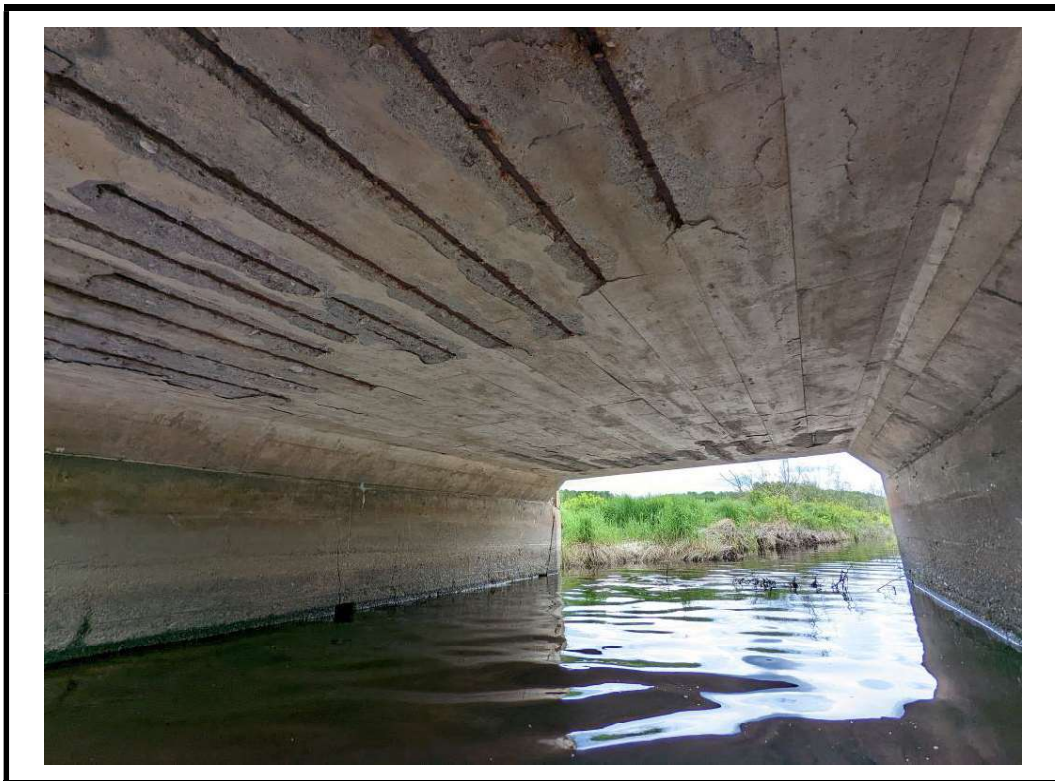
Photo 10 Spalls with exposed corroded reinforcement and severe delamination on soffit.
