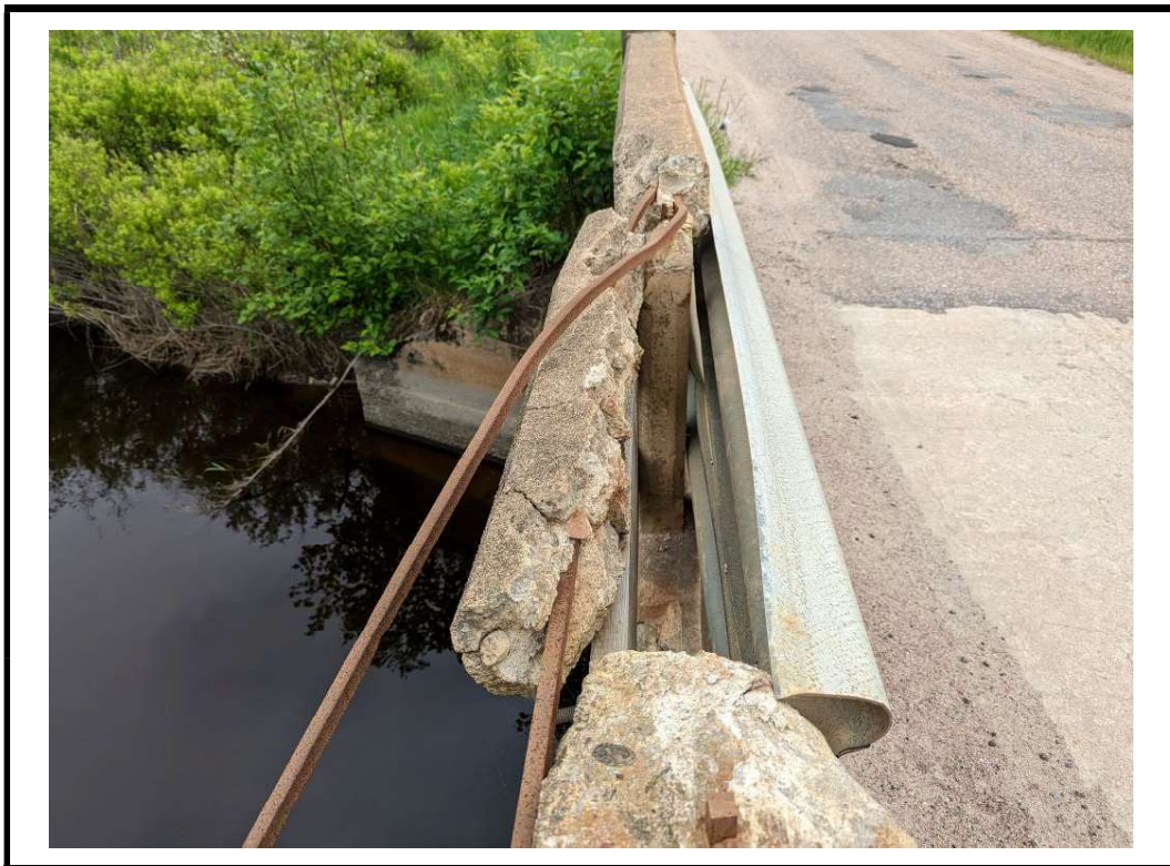
Photo 8 Exposed corroded reinforcement and steel beam on barrier
