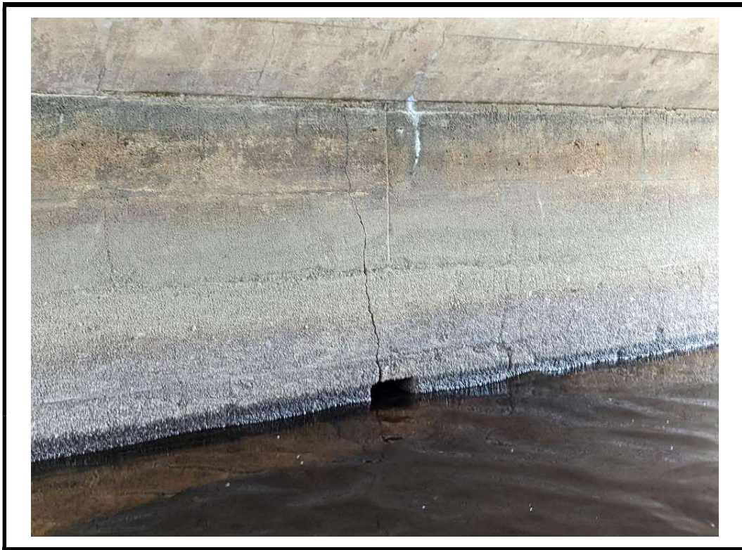
Photo 13 Medium crack with efflorescence observed on abutment wall
