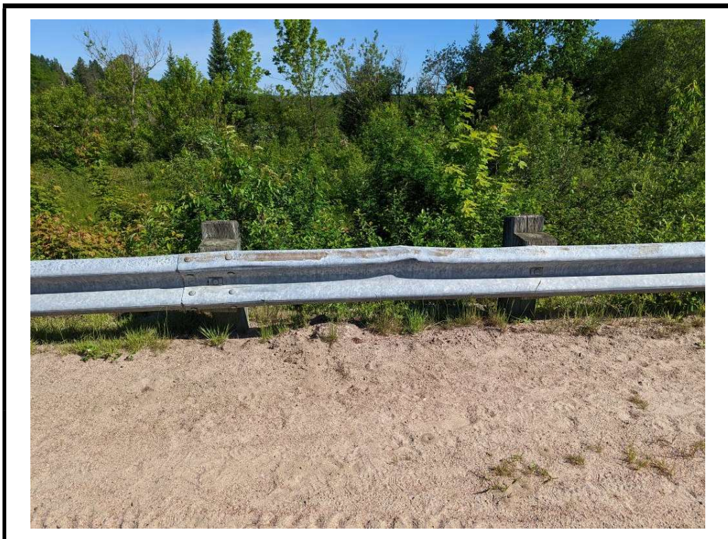
Photo 8 Collision damage noted on approach barrier at southwest corner
