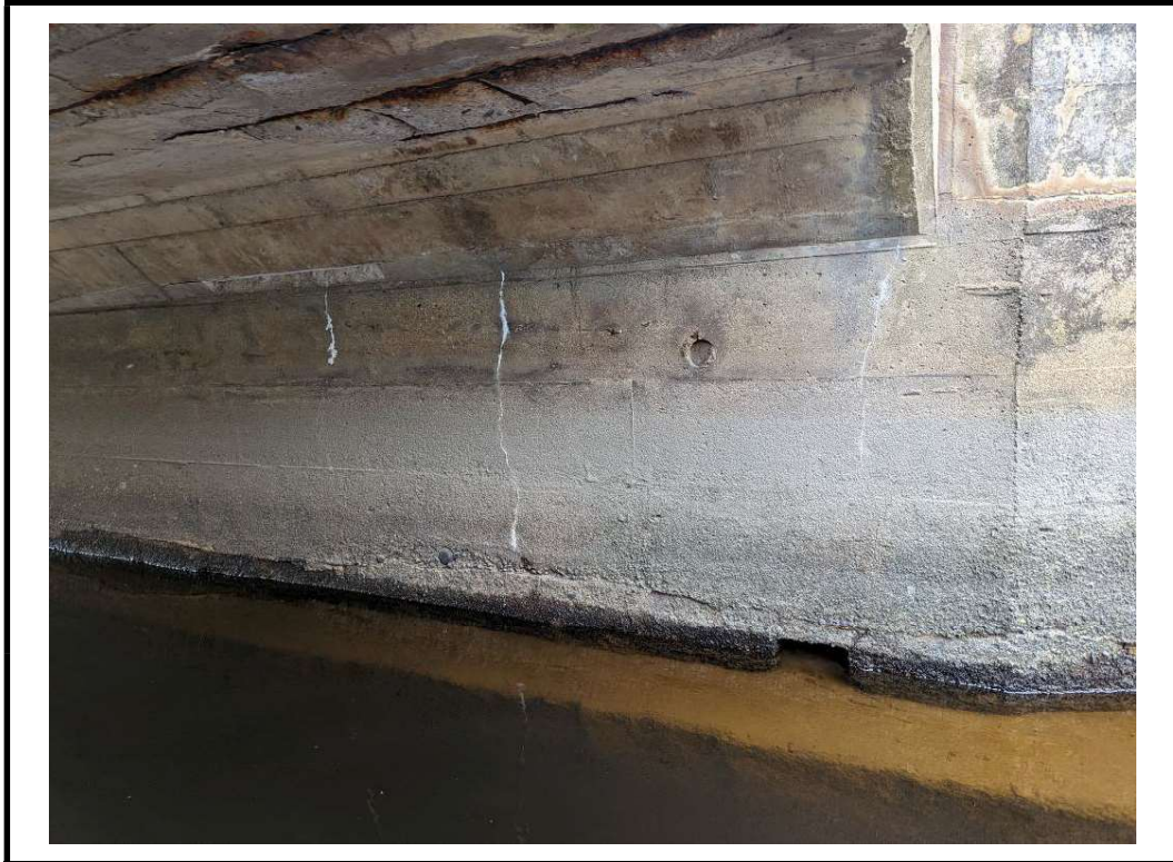
Photo 16 Moderate scaling, narrow cracks with efflorescence noted on west abutment wall
