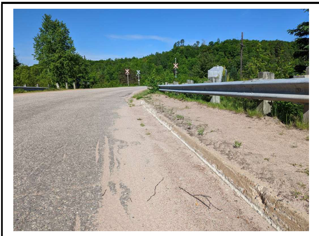
Photo 10 Significant abrasion noted on approach curb at northwest corner
