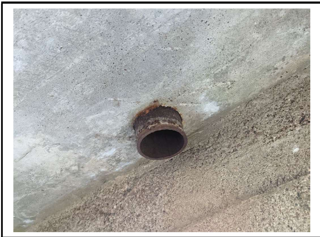
Photo 12 Corrosion and perforation noted at deck drain (Typical)
