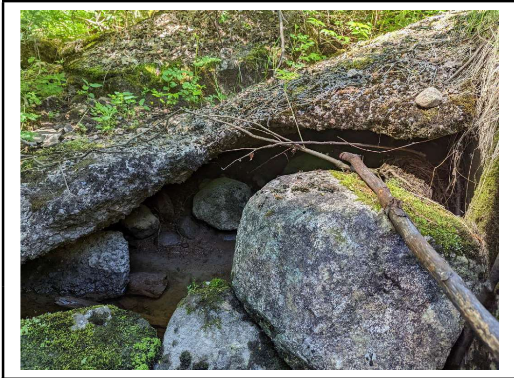
Photo 18 Concrete slope protection at southwest corner failed
