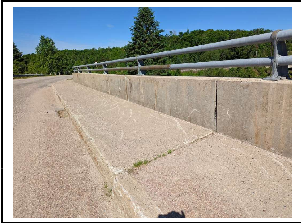
Photo 11 Narrow map cracks with efflorescence and stains with spall on parapet wall
