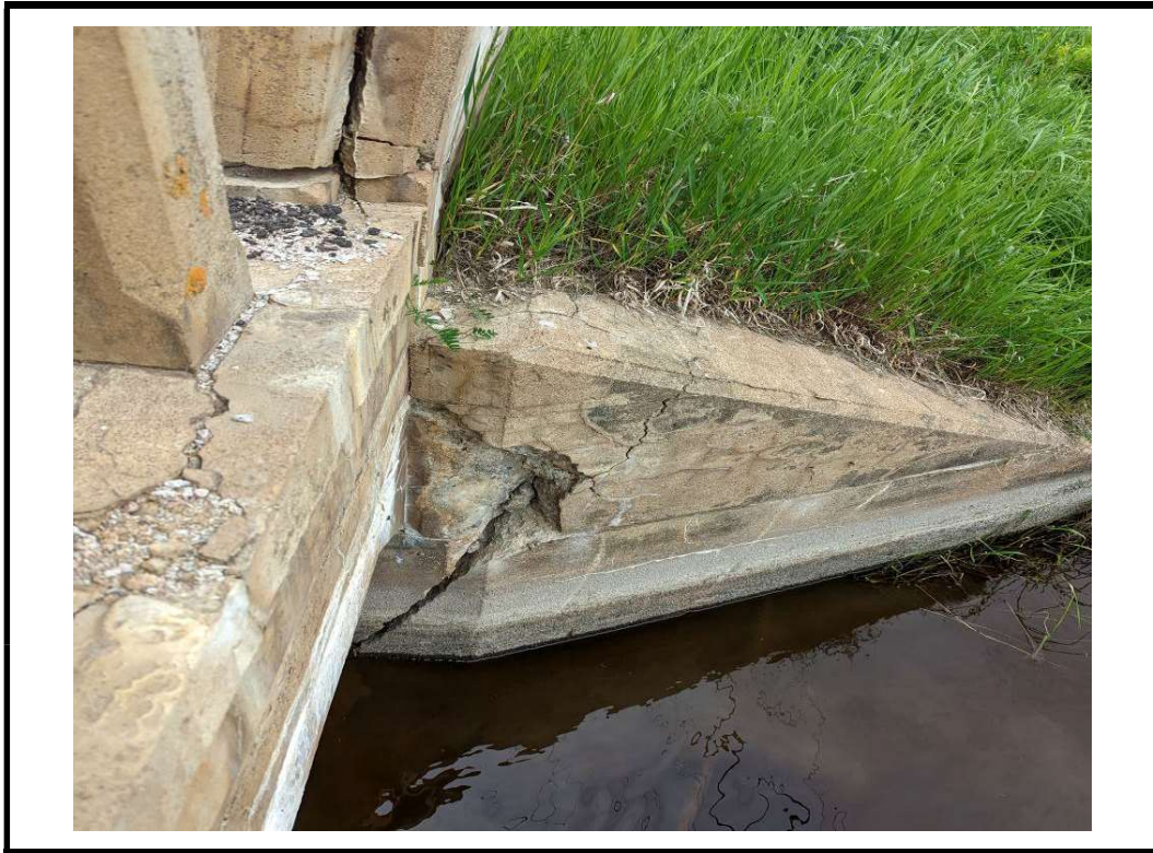
Photo 15 Large spall with crack noted on southeast wingwall
