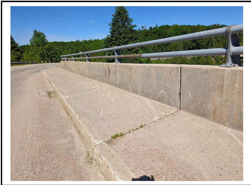
Photo 12 Narrow map cracks with efflorescence and stains with spall on parapet wall
