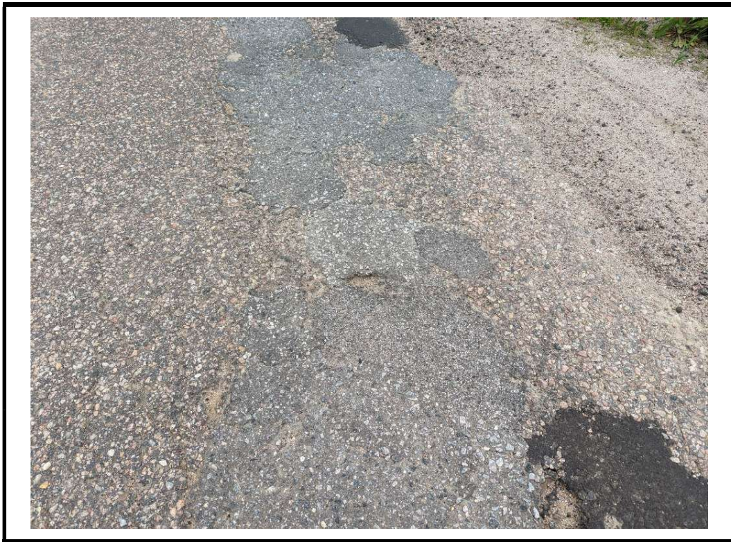
Photo 7 Asphalt patches and small pothole on west approach wearing surface
